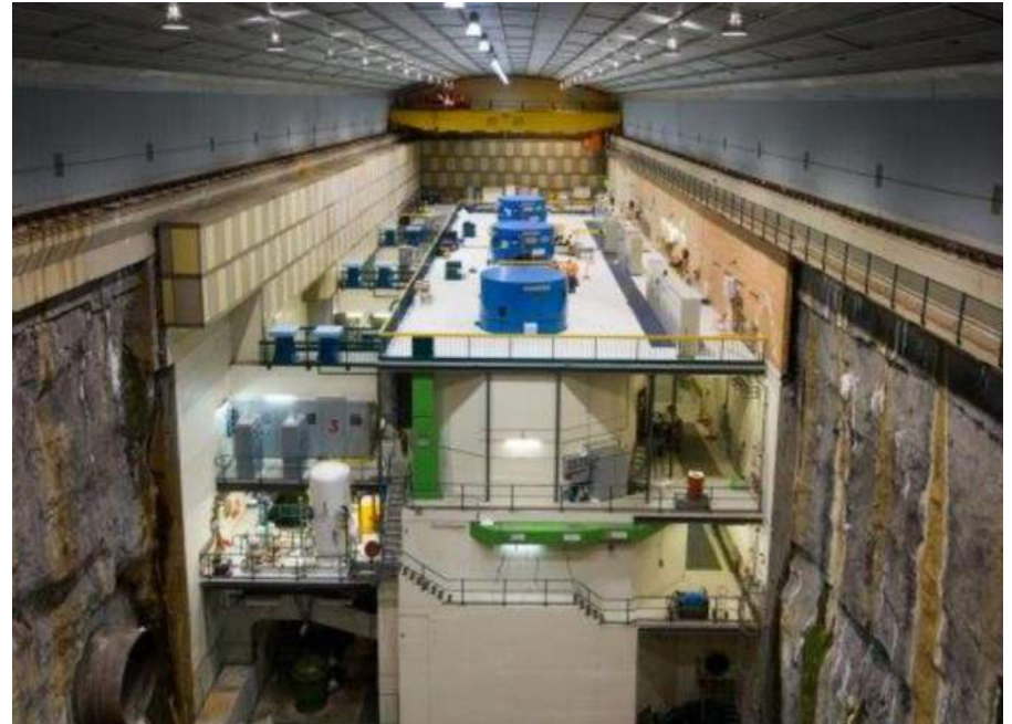
Gordon Power Station, Tasmania
